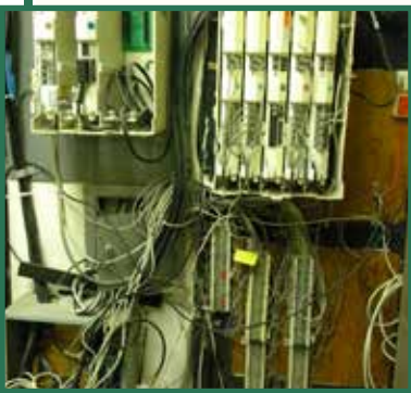
Inadequate infrastructure needs to be updated to support modern learning technology.
