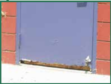
Classroom doors with dry rot need to be replaced for safety and energy efficiency purposes.
